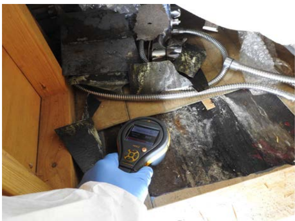
Dampness in bathroom floor
